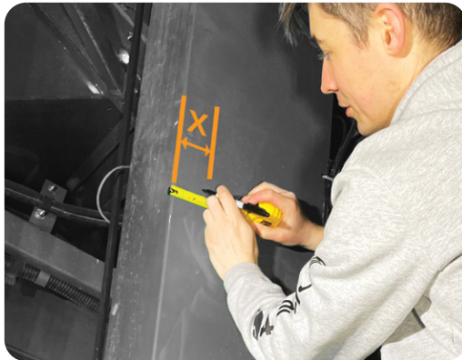
Distance (X) from the back of the clean grain elevator to the center of the drill hole
